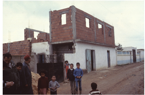
26. Housing being built incrementally along the road in Tunis. Tunis, Tunisia, circa 1984-1990.
